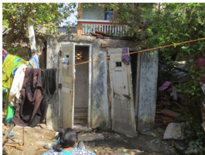
Photograph 4: Toilet doors in a house damaged during 2006 floods and still being used in the same state at Moti Ved
