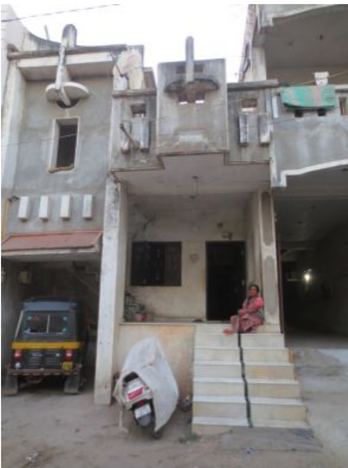
Photograph 8: Raised plinth (4'-6") of a house constructed after an earlier flood, in an elevated hamlet at Bhesan. Notice a deep empty hall on the ground floor of the house on right; The family lives on the first floor
